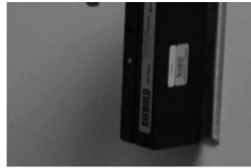
Fig. 1.29 An Access Card Security System
