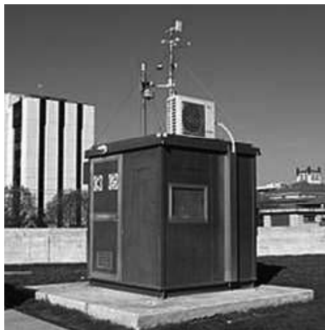
Fig. 4.8 Air Quality Monitoring Station
